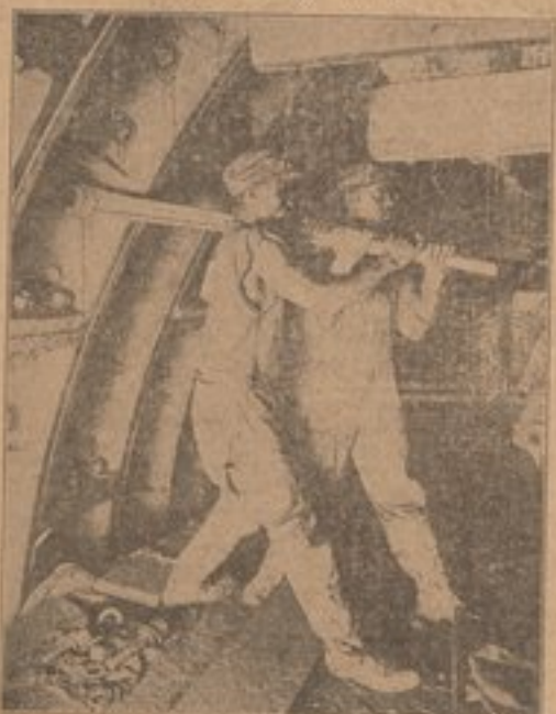
At work in the city tunnel in Chattanooga. These workers get 25 cents an hour, under unbearable speed-up, working sometimes at a 25-hour stretch. "If you don't like," says the boss, "get out." Workers fall from exhaustion at the end of the day's work. Organization and struggle is the only way out.
