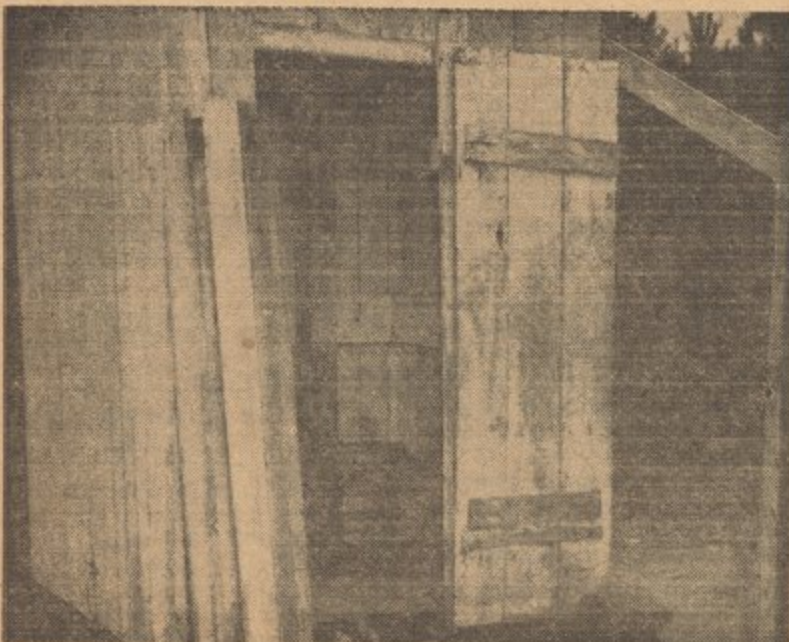
IT'S FACILITIES like this "toilet" in a Negro school in South Carolina that are responsible for the demand for an end to Jim Crow education.
