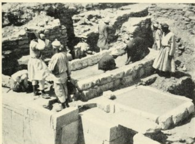
FIG. 15. PREPARING TO REMOVE UPPER COURSES OF DECORATED CHAMBERS, WHICH ARE FILLED WITH SAND TO PREVENT THE COLLAPSE OF THEIR WALLS
