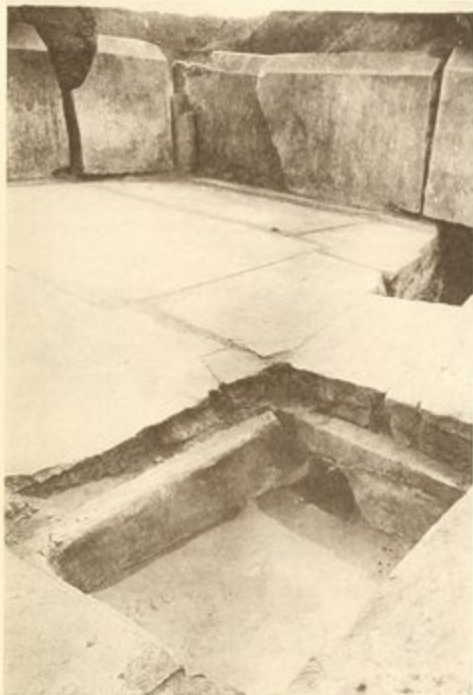
LEAD TANK OF DRAIN
