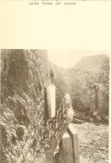
STONE LINING PARTLY FALLEN FORWARD.
